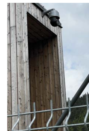
Instalace kamer DS-2DF8C442IXS-AEL(T5)
